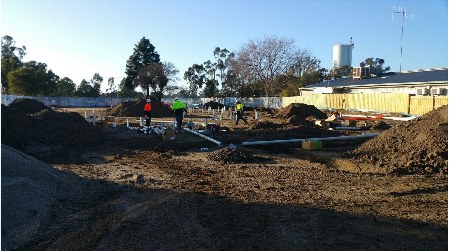
Above: Construction workers are installing the underground services needed for the Barham Multipurpose Service (MPS). The next step is the concrete pour for the main MPS facility.
